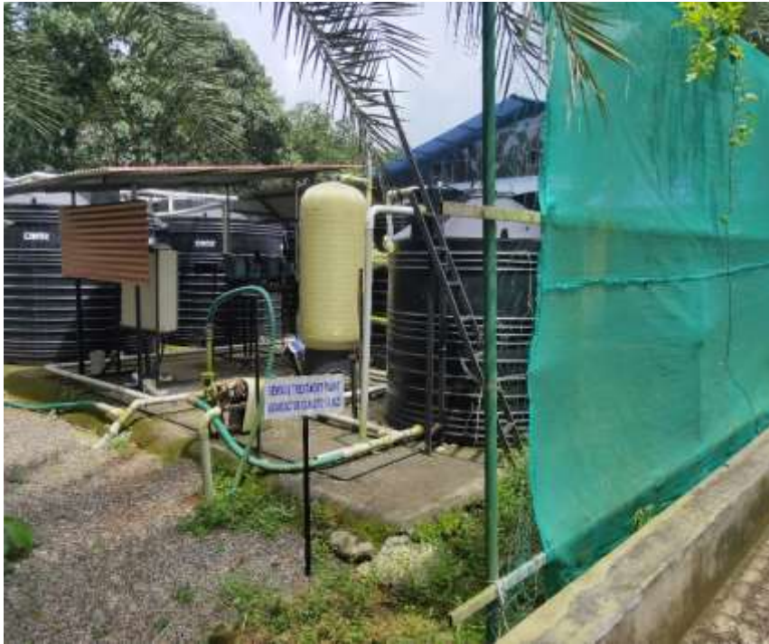
Figure 6 SEWAGE TREATMENT PLANT
