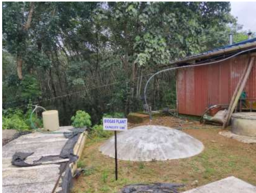
FIGURE 3: BIO GAS PLANT
